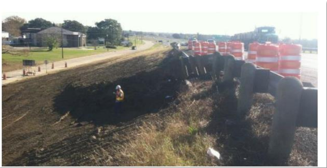
Figure 19 Failure at Beaumont site, before construction of soil nail wall.
