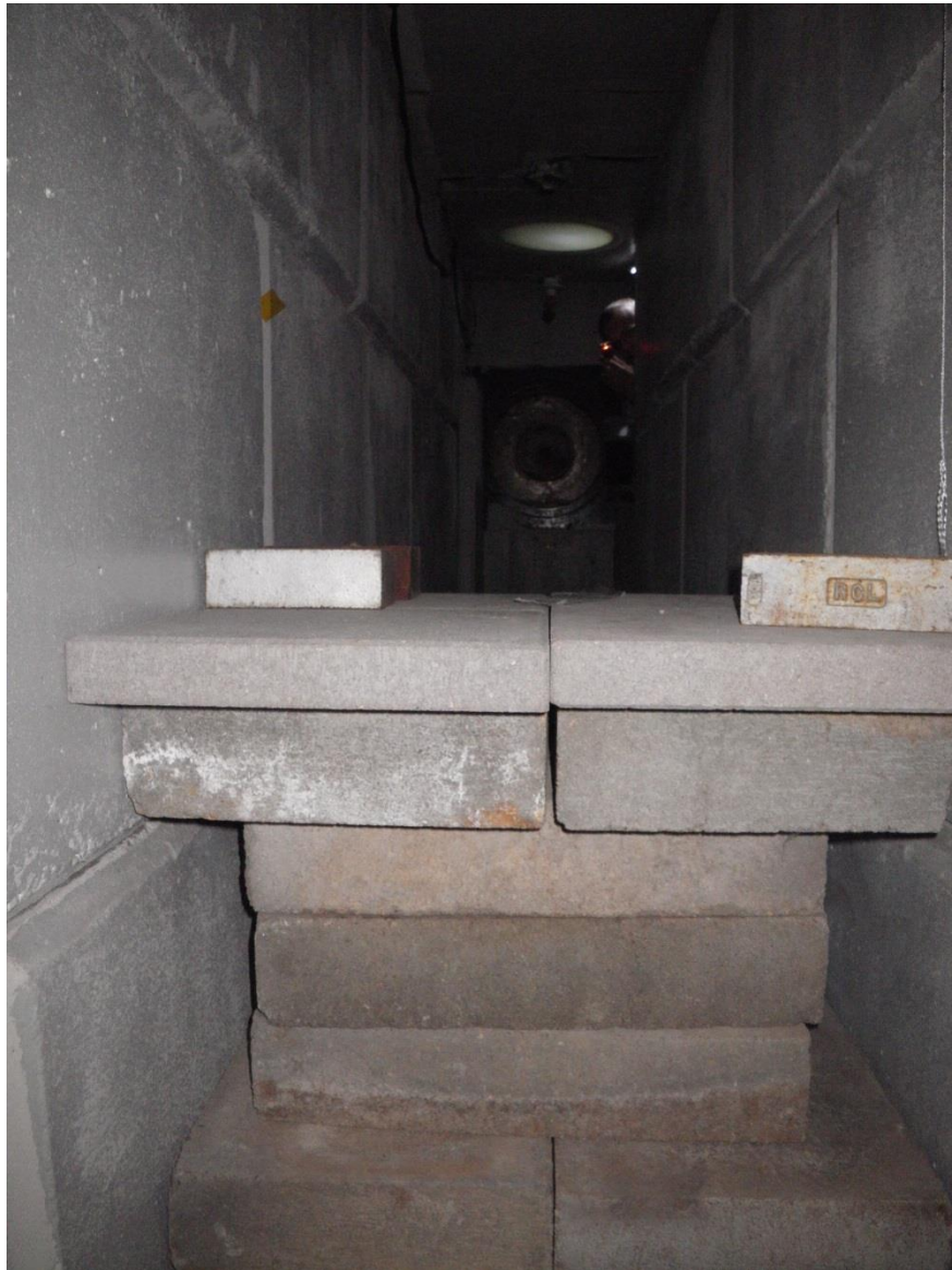
Figure 40. Hydraulic vertical lift support blocks.
