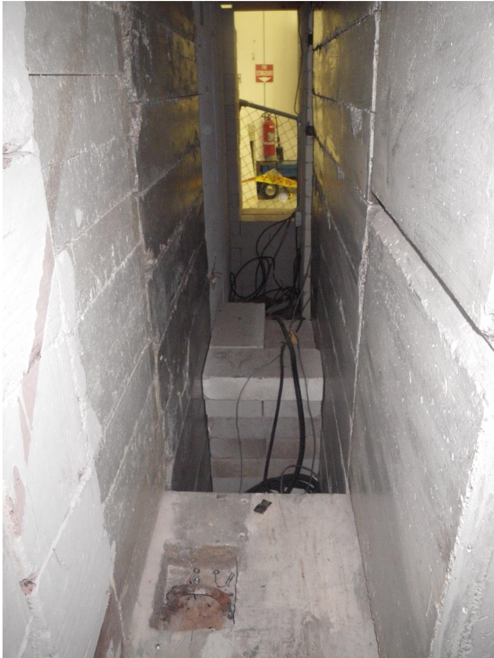
Figure 43. View from inside the perpendicular portion of the cave after the removal of the film tray and trolley track rack.
