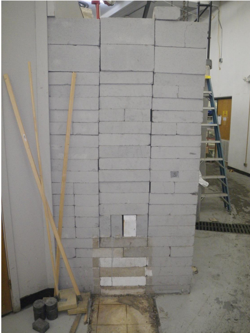
Figure 42. Portion of the shielding wall that was removed to allow the removal of the neutron radiography film tray and trolley track rack.
