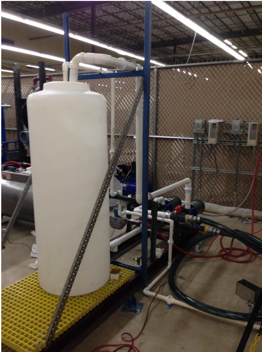
Fig. 16—Skid for the Pumps and Mud Tank
