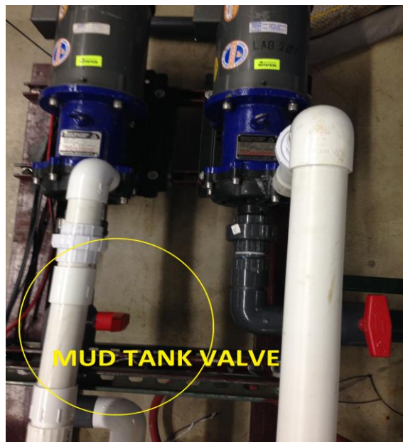
Fig. 56 – Mud Tank Valve
