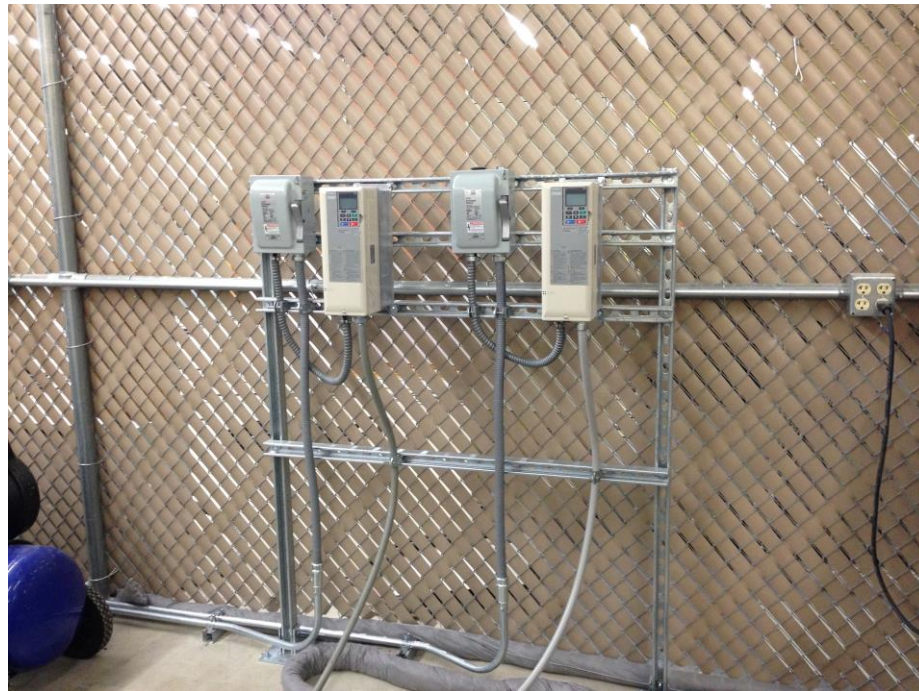
Fig. 15—Variable Frequency Drives (VFD)
