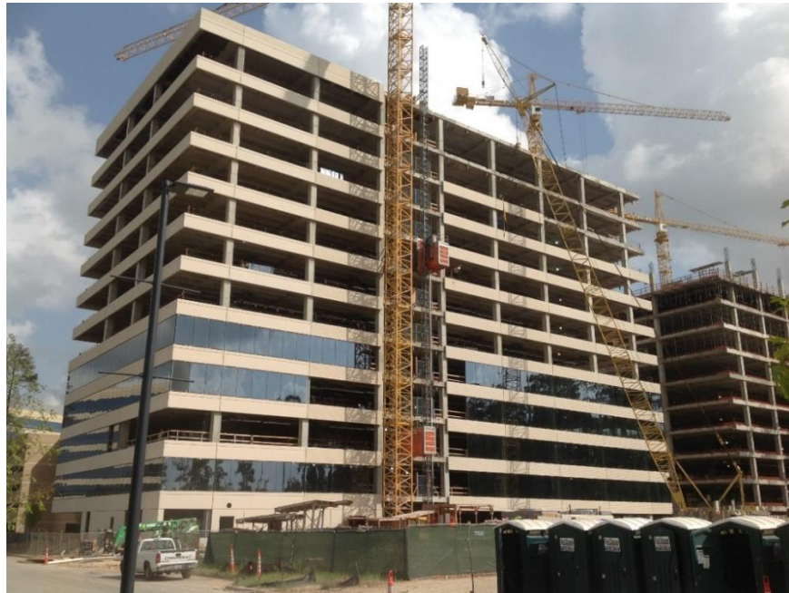
Figure 31. The progress of the curtain wall installation at the South façade. Image: Andres Martinez, dated August 18, 2014.
