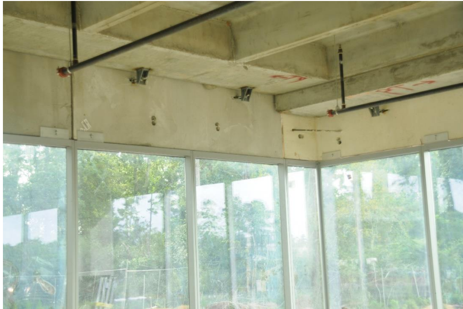
Figure A-5. Evidence of removed curtain wall anchor clips at 4 th floor, Southeast corner. Picture 4a. Image: Andres Martinez.
