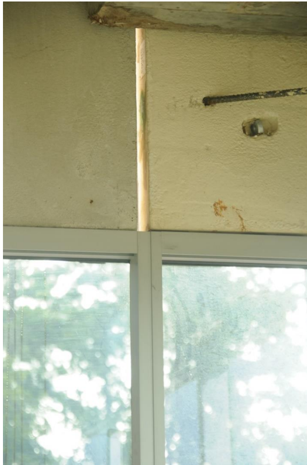
Figure A-7. Interior view of Joint misalignment between cladding systems. Picture 5. Image: Andres Martinez.
