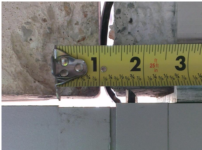
Figure A-12. Detail of horizontal misalignment between curtain wall and precast panels. Picture 6b. Image: Andres Martinez.
