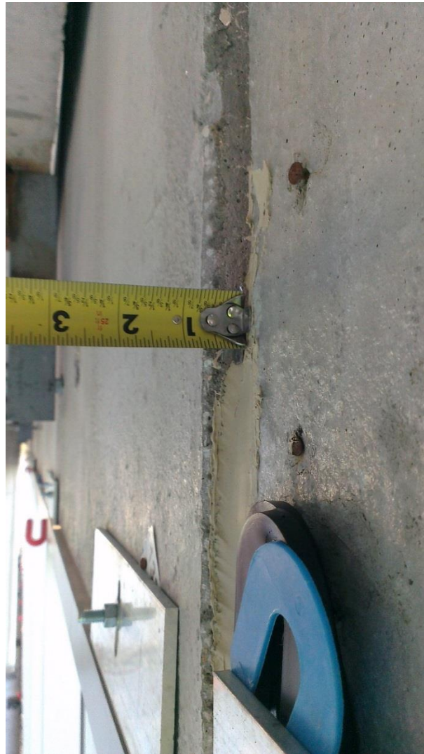
Figure A-3. Tolerance discrepancies between curtain wall anchor clips and precast panels. Picture 3a. Image: Andres Martinez.
