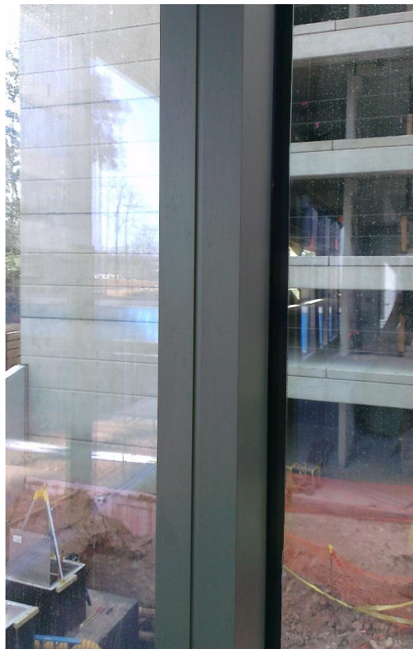
Figure A-14. Interior view of custom aluminum cover displaced at the exterior of the building. Picture 10. Image: Andres Martinez.
