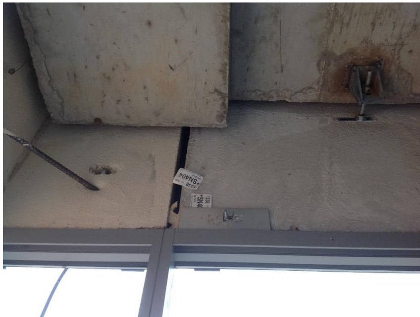
Figure A-8. Interior view of joint misalignment between cladding systems at building corner. Picture 8b. Image: Andres Martinez.
