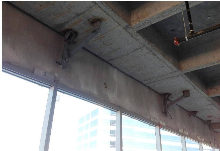
Figure A-4. Evidence of removed curtain wall anchor clips at 3 rd floor, West façade. Picture 3b. Image: Andres Martinez.
