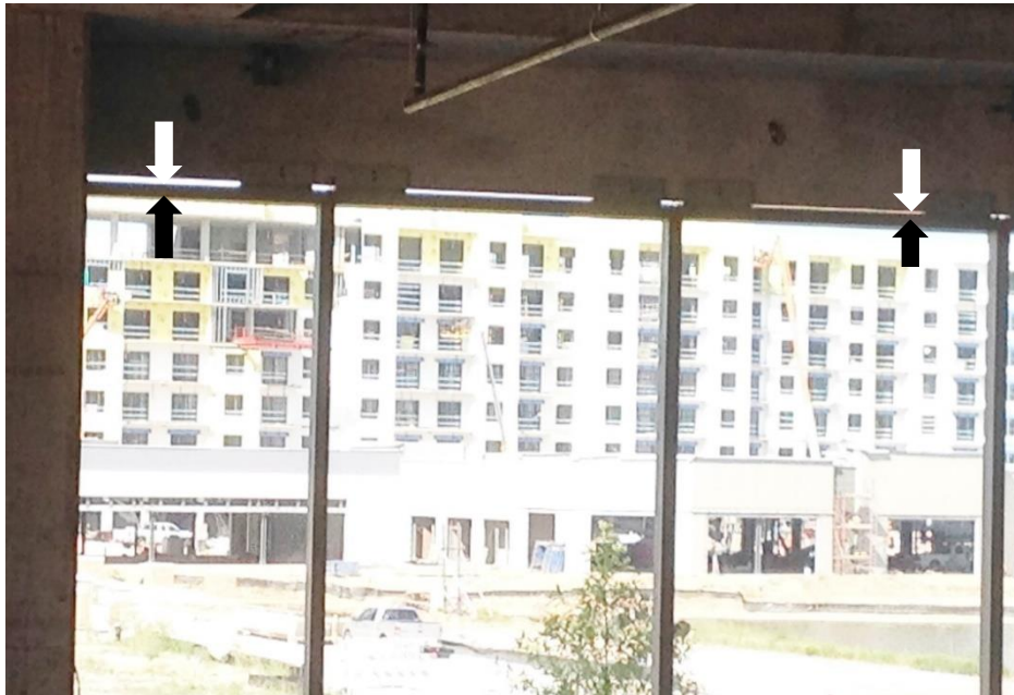
Figure 35. Tolerance issues at the top of the curtain wall panels. East façade, interior view. Image: Andres Martinez.
