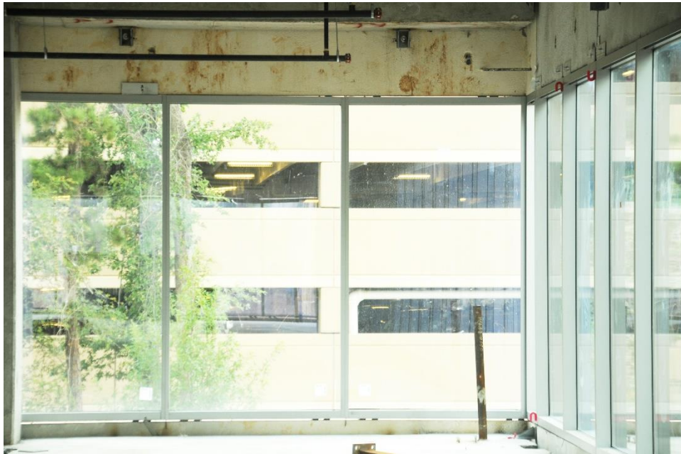
Figure A-6. Uneven precast panels at top of curtain wall panel. Picture 4b. Image: Andres Martinez.
