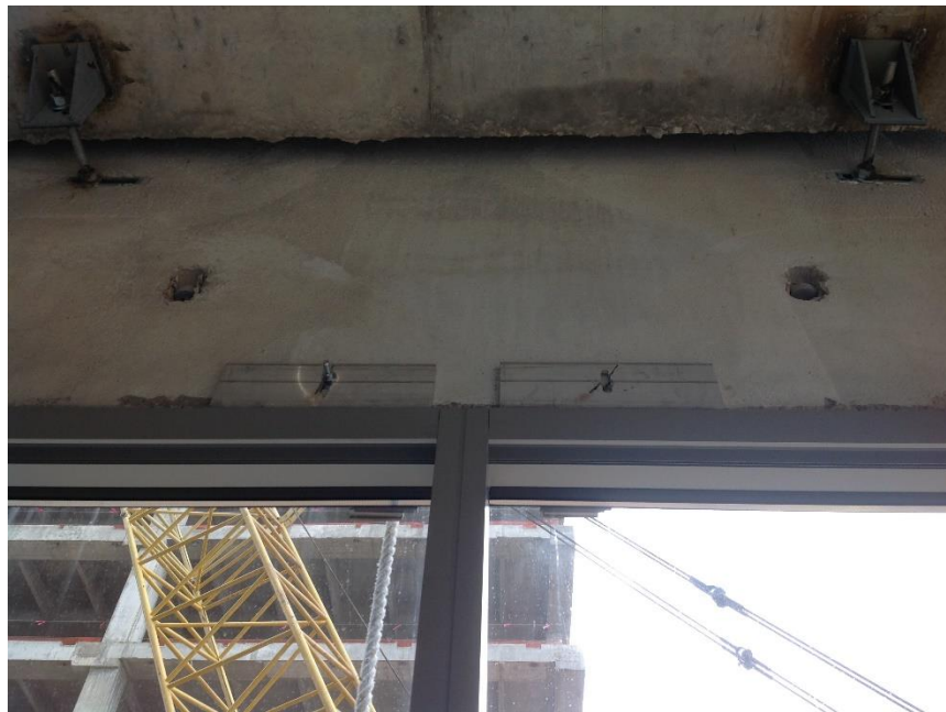
Figure A-13. Alteration of curtain wall anchor clips. Picture 8a. Image: Andres Martinez.
