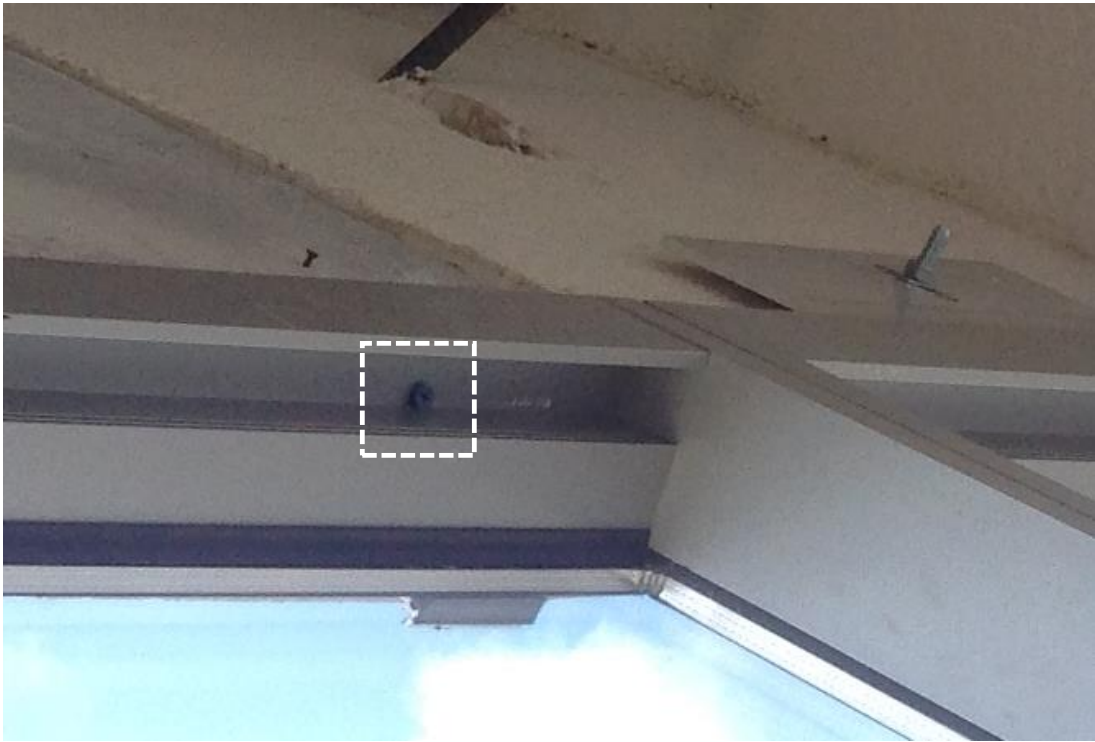
Figure 37. Detail of curtain wall panel screwed through the blind pocket. Image: Andres Martinez.
