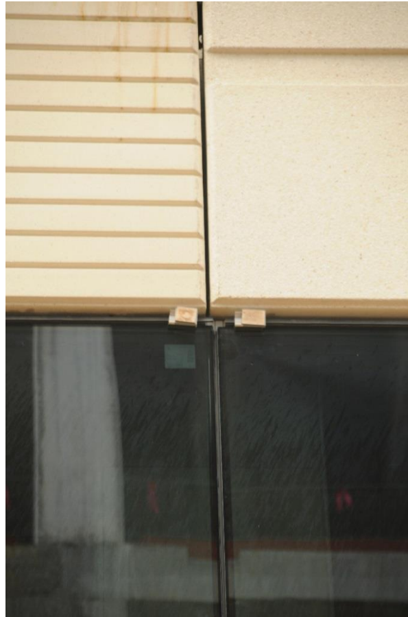
Figure A-2. Misalignment between precast and curtain wall panels joins at East façade. Picture 1b. Image: Andres Martinez.
