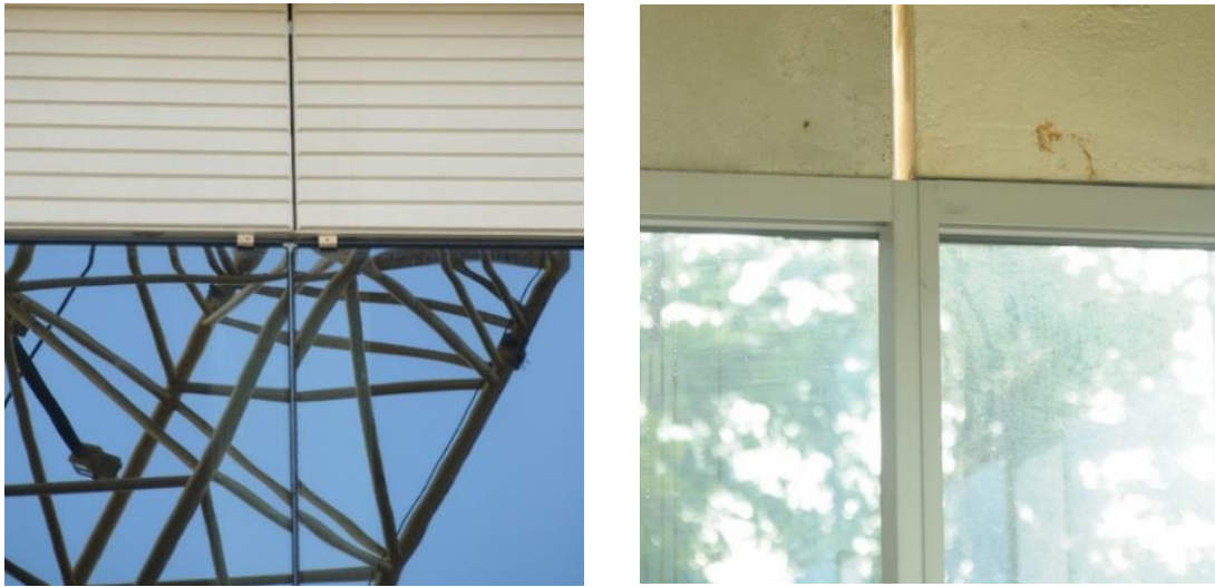
Figure 38. Misalignment of the curtain wall and precast panel joints. Exterior view of at the North façade (left), interior view at West façade (right). Image: Andres Martinez.
