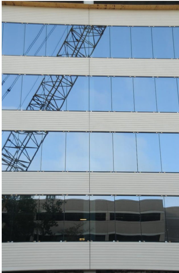
Figure A-1. Alignment of precast and curtain wall panels at North façade. Picture 1a. Image: Andres Martinez.
