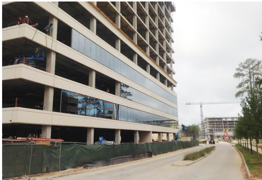
Figure 30. The progress of the curtain wall installation at the North façade. Image: Andres Martinez, dated July 28, 2014.
