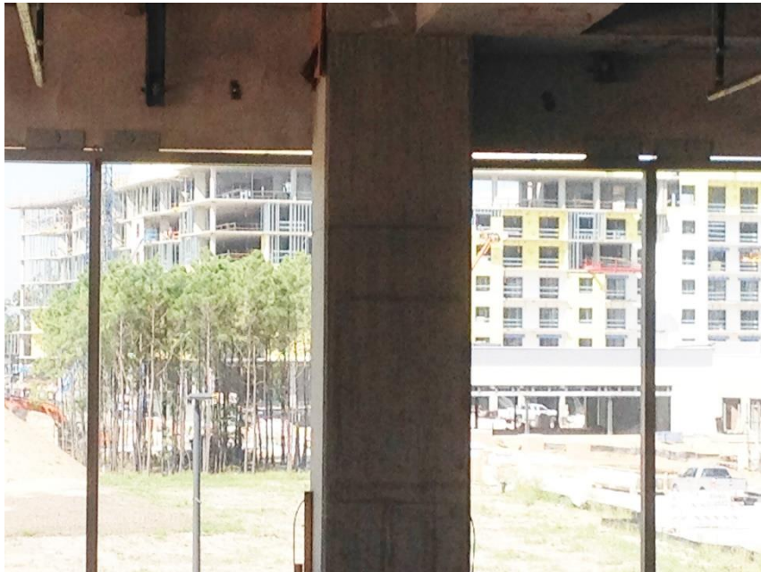
Figure A-10. Tolerance discrepancies between cladding systems and top of the curtain wall panels. Picture 9. Image: Andres Martinez.
