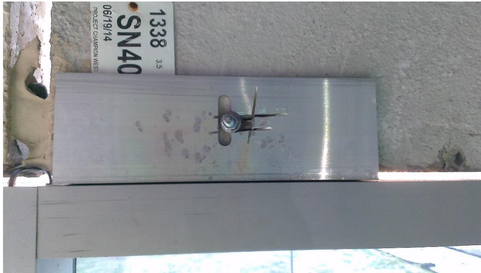
Figure A-9. Alteration of curtain wall anchor clip caused by horizontal displacement of the panel. Picture 8c. Image: Andres Martinez.
