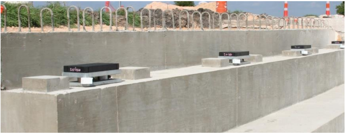
(b) North End Load Cell Assembly
