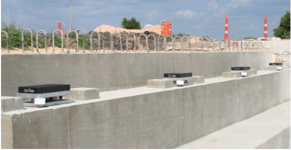
(a) North End Load Cell Assembly
