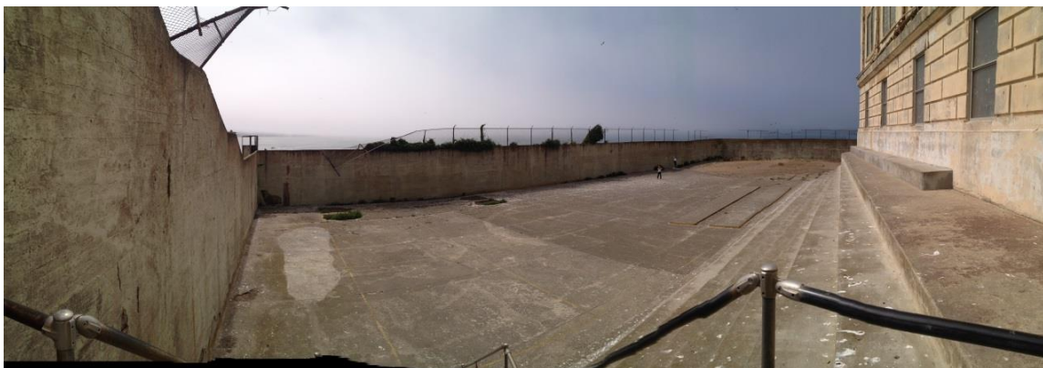
Figure 2 Recreational yard: Damage and Repair (Manrique 2013)
