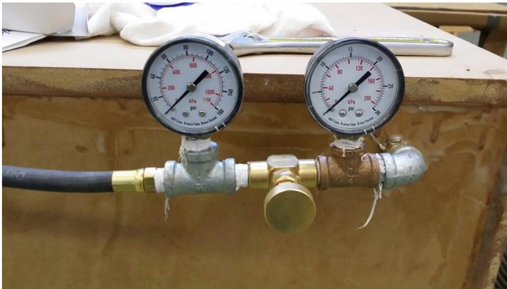
Figure 13. Pressure gauges and needle valves
