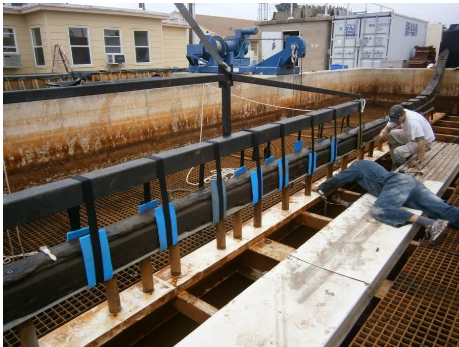
Figure 10.29. CRL graduate student staff make final adjustments in preparation for raising the keel skag and completing the disassembly process. Photograph courtesy Conservation Research Laboratory.
