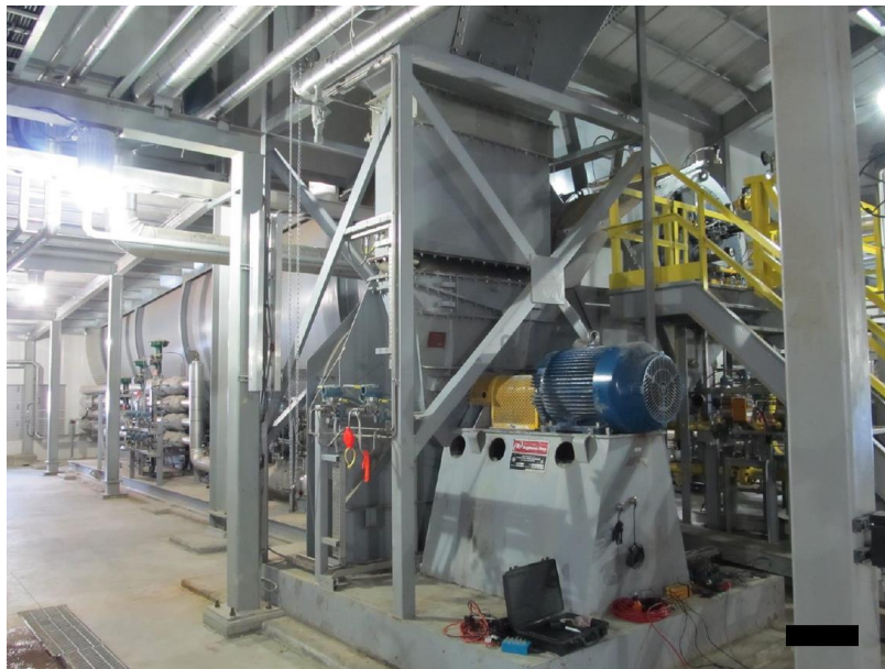
Fig. 22 Machinery train driven by VFD
