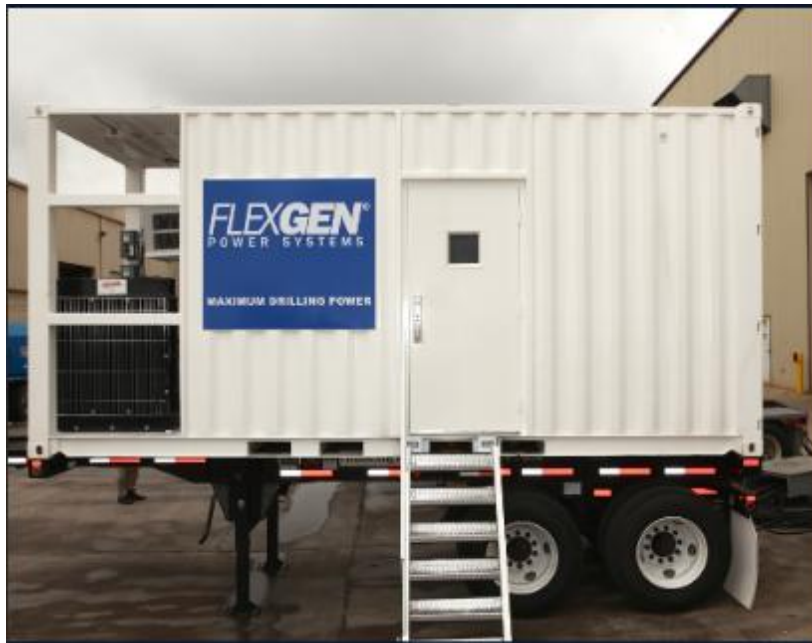
Figure 10: FlexGen ultracapacitor system
