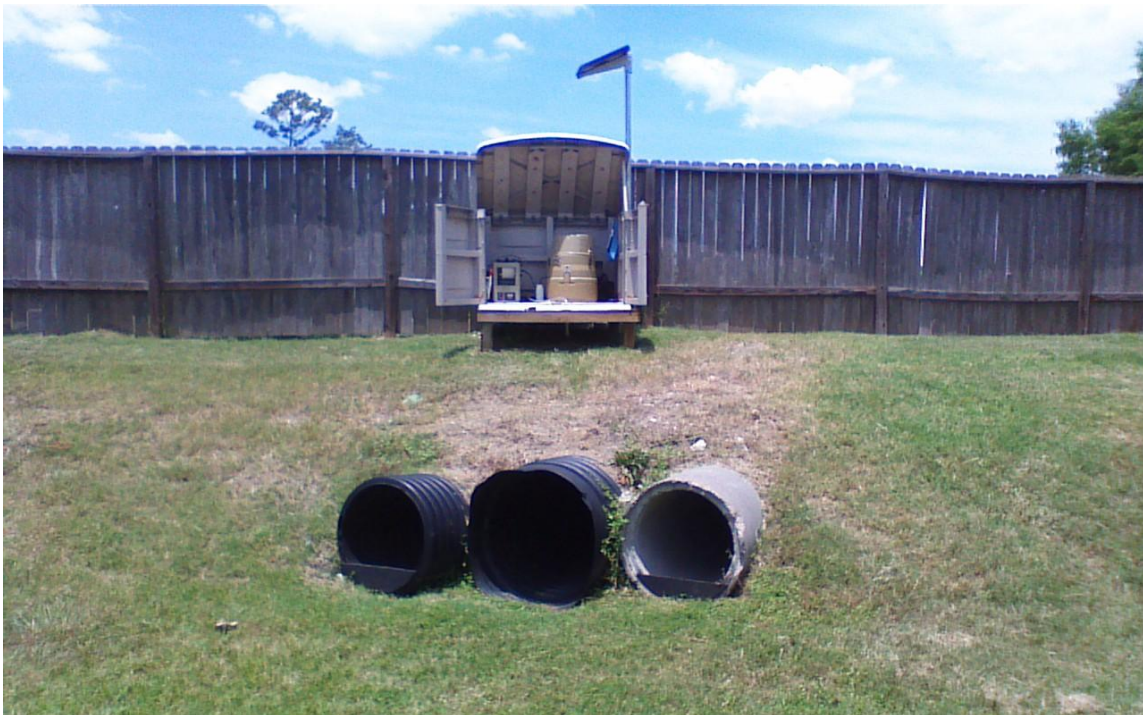
Figure 7. Detention basin used to collect runoff from the control site. All instrumentation is kept inside of a storage box on the apex of the basin.
