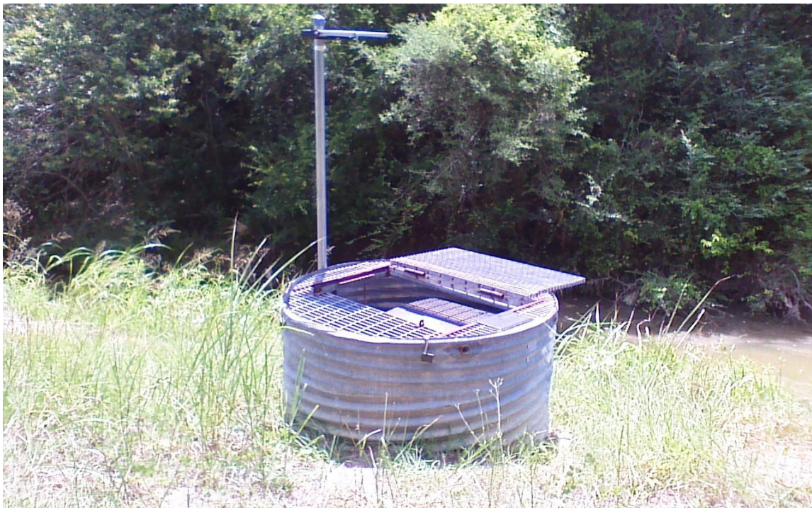
Figure 6. Manhole used for equipment storage and runoff collection at the OSSF site.
