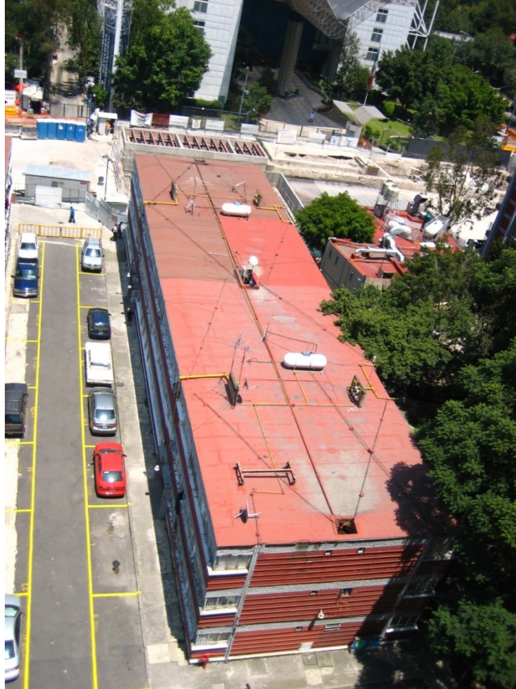
Figure 55. Liquefied Petroleum (LP) Gas Tanks Located on the Rooftop of One of the Small Three-Story Buildings in the Complex. (Photo by Jose Luis Bermudez Alcocer).
