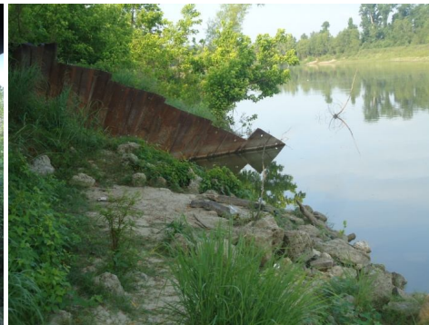
b. Failed sheet pile
