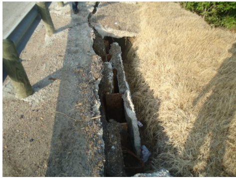
a. Sheet pile inside the crack
