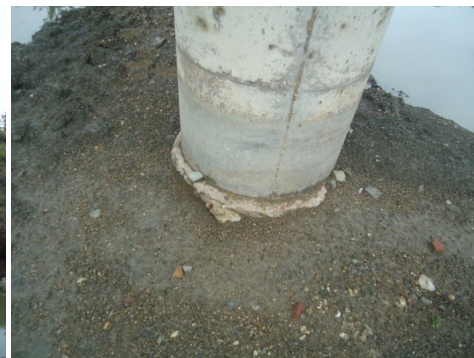
d. Column exposed
