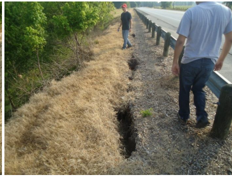
b. Crack next to the road
