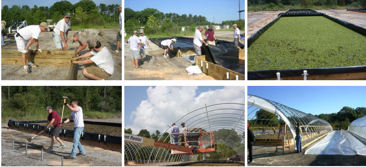
Clockwise from top left: CISE, TPWD and local volunteers: constructing weevil rearing tanks, installing pond liners, filled tanks, driving greenhouse legs, erecting greenhouse frames, installing greenhouse skin
