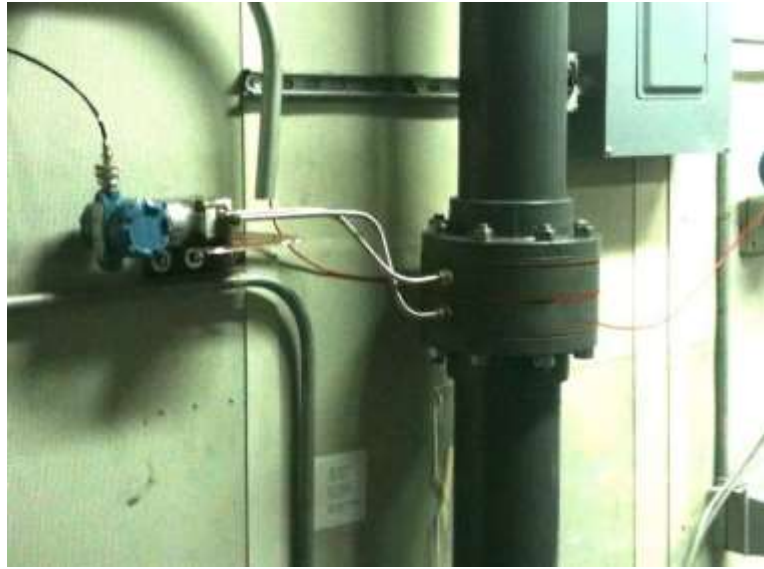
Figure 52. Orifice Flow Meter [24]
