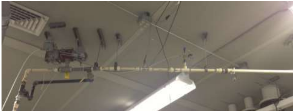
Figure 55. Air Supply Setup
