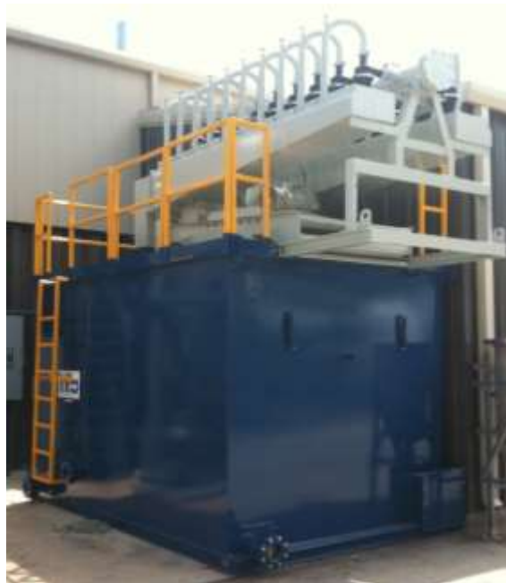
Figure 46. Tank and Separator Assembly
