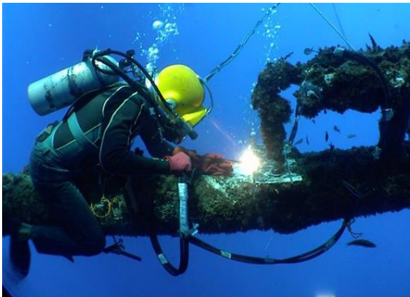
(e) A diver doing repair work on a marine structure with marine growth (Subsea Explore Services, 2013)
