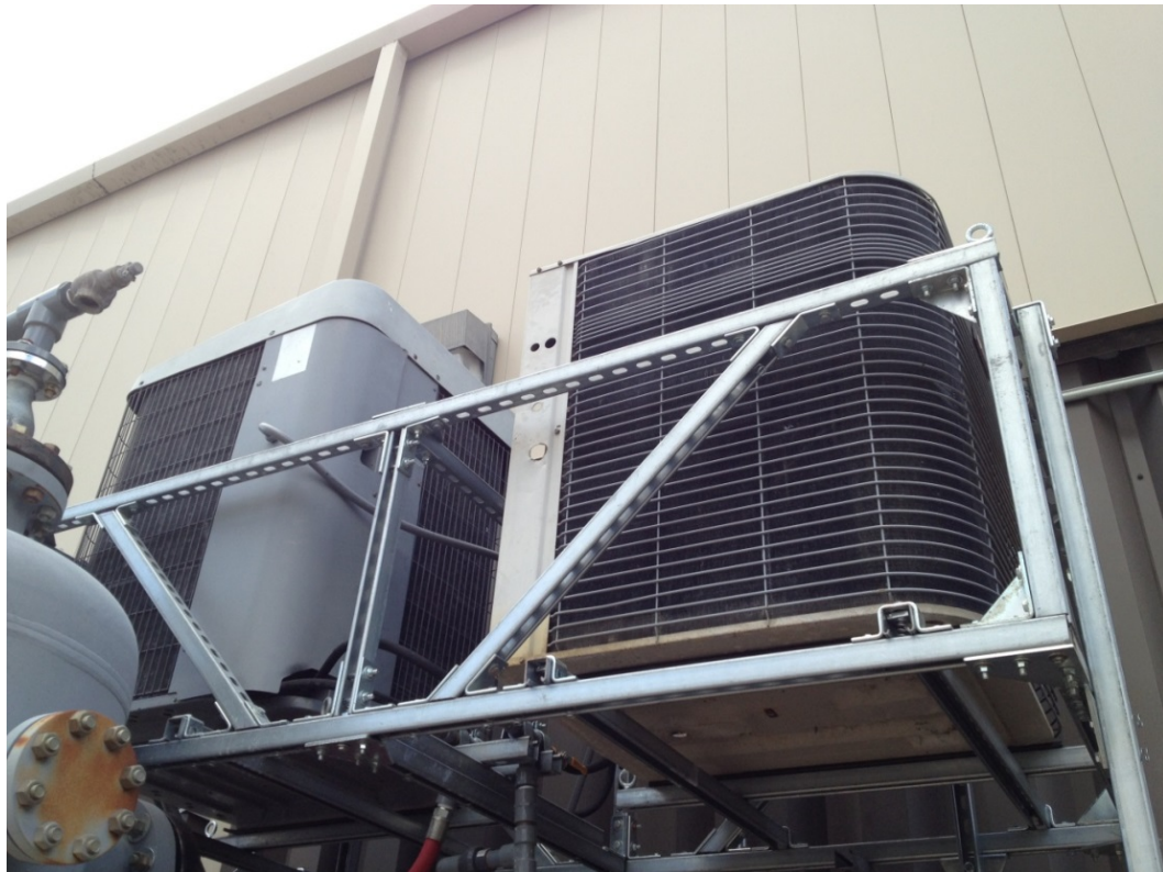
Figure 11: Heat exchangers and support structure
