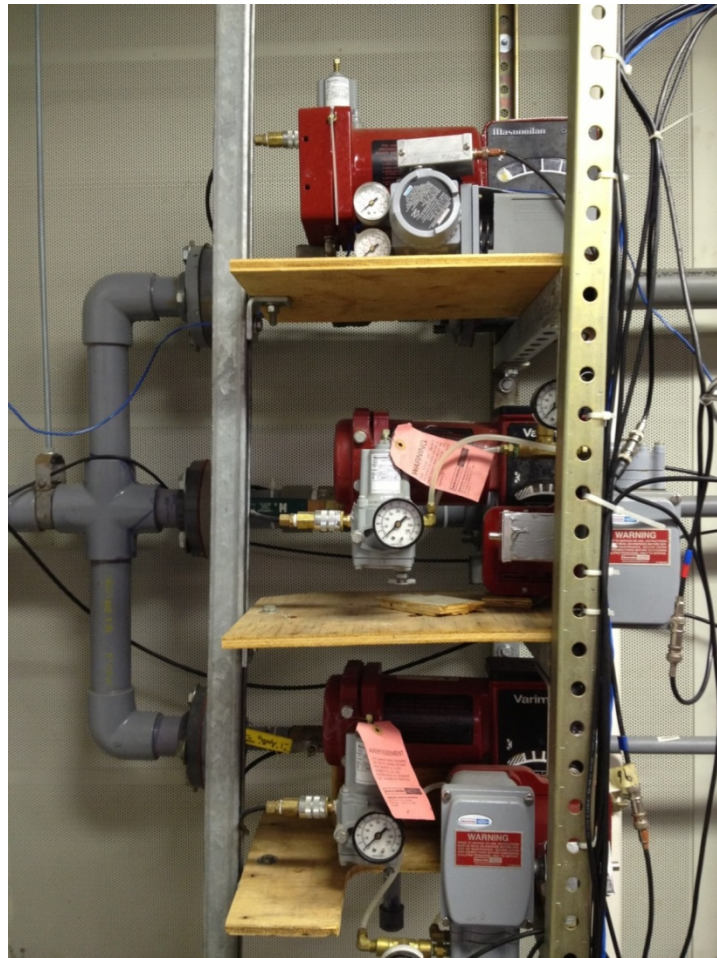
Figure 13: Water flow control valves
