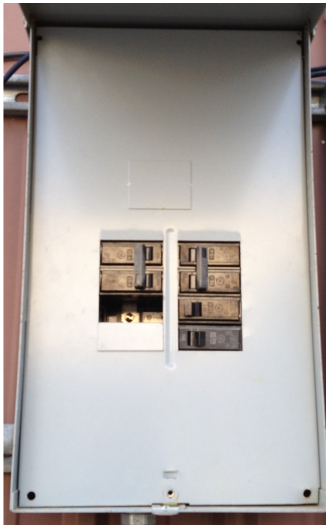
Figure 29: Circuit breaker for heat exchanger fans
