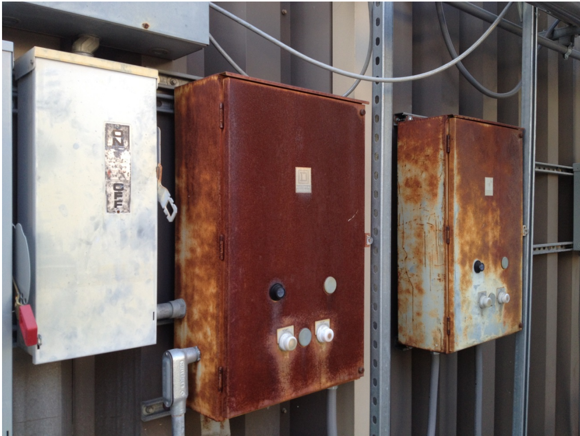
Figure 30: Circuit breaker and motor starter for circulation pump
