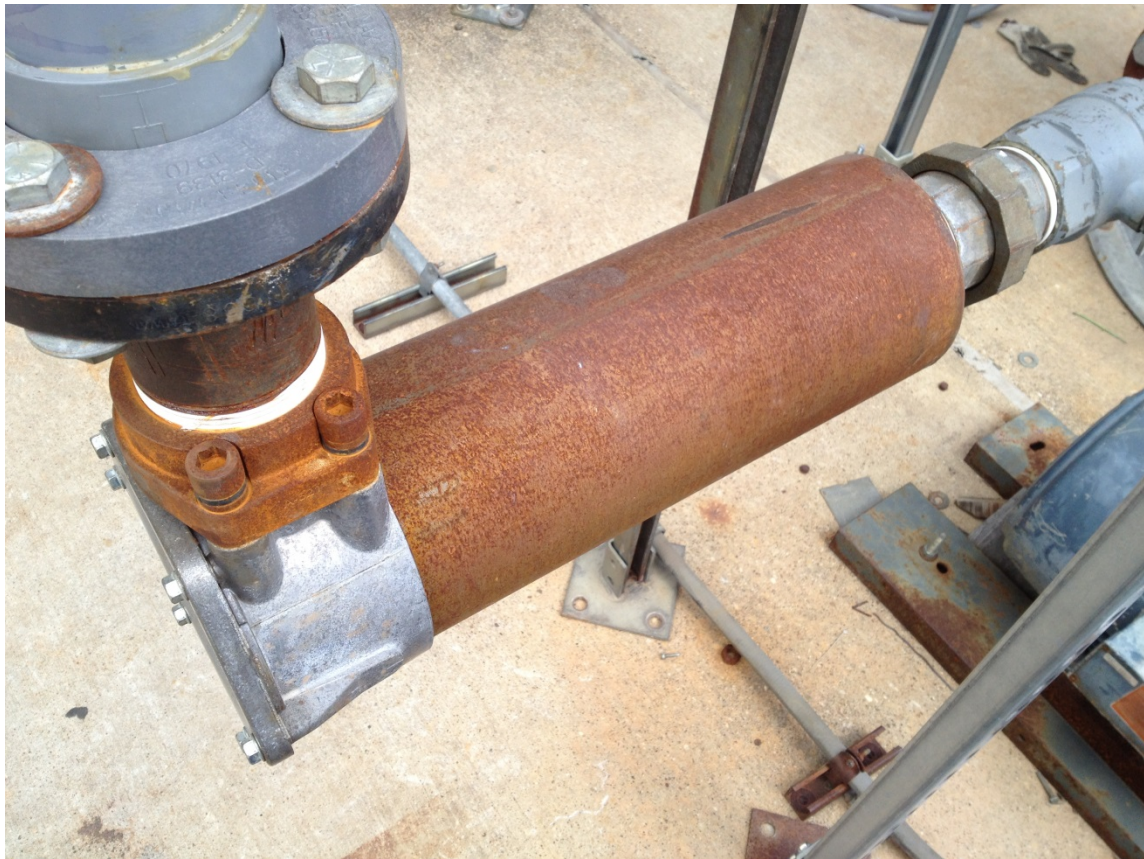
Figure 10: Main water filter
