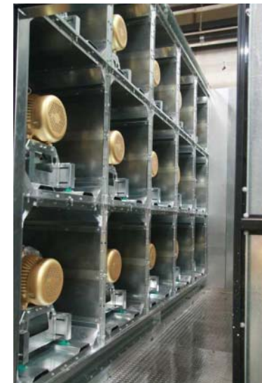
Fanwall AHU (TRIP)
