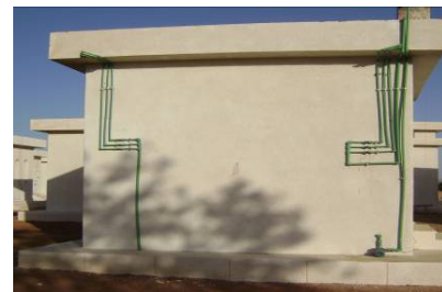
(c). Room with active concrete
