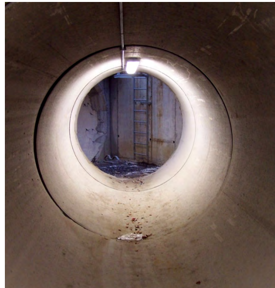
Figure 3.2. Earth tube installed in Nursing Library building
