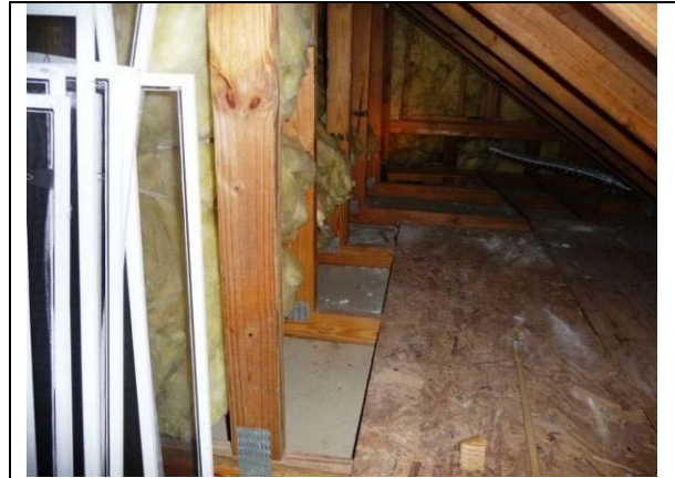
Figure 1 View of kneewall and main floor space (far), and bonus room wall and floor cavity (left).
