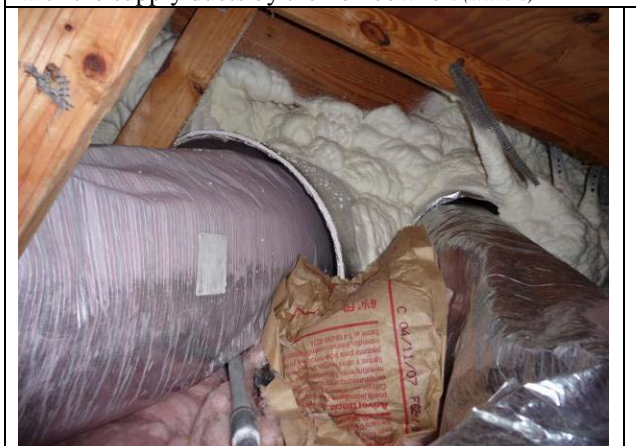
Figure 5 East side floor cavity isolated from the garage attic; a protective vapor barrier/thermal barrier sleeve isolates the foam from the exterior of the supply ducts to reduce the condensation potential. (Withers)
