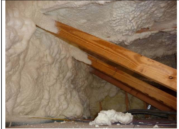
Figure 21 Foam applied to wall and ceiling of the bonus room floor cavity (3' high). (Withers)
