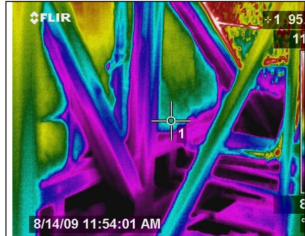
Figure 7 IR view inside the attic shows cool temperatures in the floor space and cooled surfaces low in attic. (Withers)
