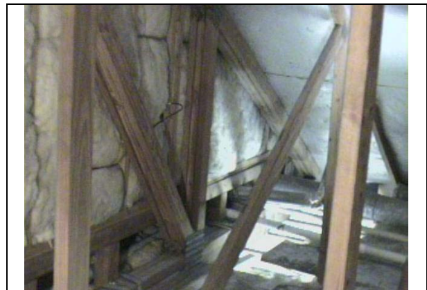
Figure 8 Photo of IR image above. The floor cavity at the bottom of the wall is open to garage attic. (Withers)
