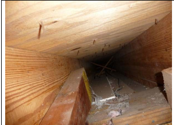
Figure 14 View from soffit vent looking inside towards floor space in area having no batts. (Withers)
