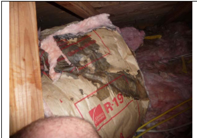
Figure 4 Moisture condensed on flex ducts and accumulated on insulation materials placed in contact with the supply ducts by the homeowner. (Withers)
