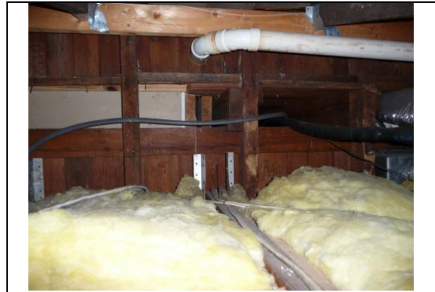
Figure 24 Floor cavity connected to attic space before repair. (Withers)
