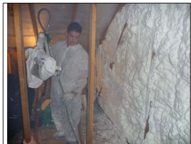
Figure 9 Technician finishes up kneewall and floor cavity insulation/air tightening. (Photo credit Ian LaHiff)
