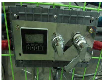
Figure 4 Temperature control box
