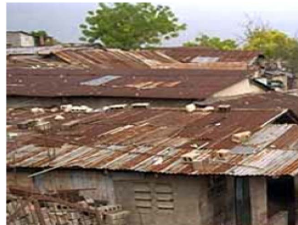
Figure 20. Metal Roofs Corrosion, Port-au-Prince
