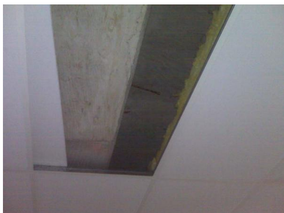
Figure 2. Insulation not present along column, but present in most of parking garage drop ceiling.
