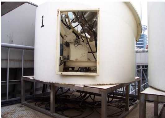
Fig. 3 Corrosion of the body
