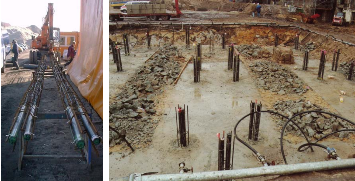
Figure 2: pipes fixed at the reinforcement of two energy piles (on the left), pipes and reinforcement fitted-in the foundation (on the right)
