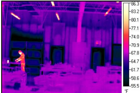
Figure 3. Thermal Image of Annex Studio (Note: Thermal image taken during cold weather)
