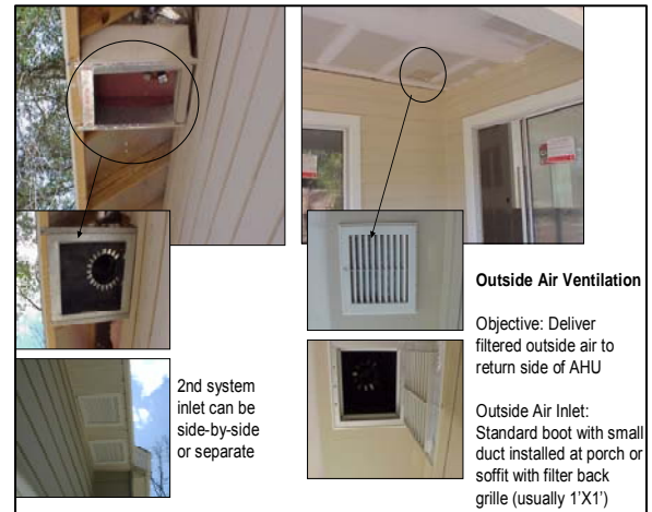
Figure 2. Details of the WHMV system installed in over 500 residences in Gainesville, FL since 1999 without any reports of occupant complaints.
