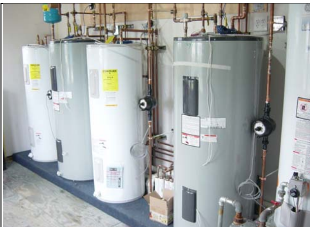
Figure 7. One half of the tanks inside the test shed.
