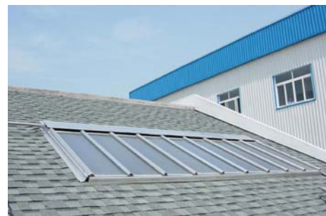
(b) Integration of solar collectors with asphalt shingle roofing
