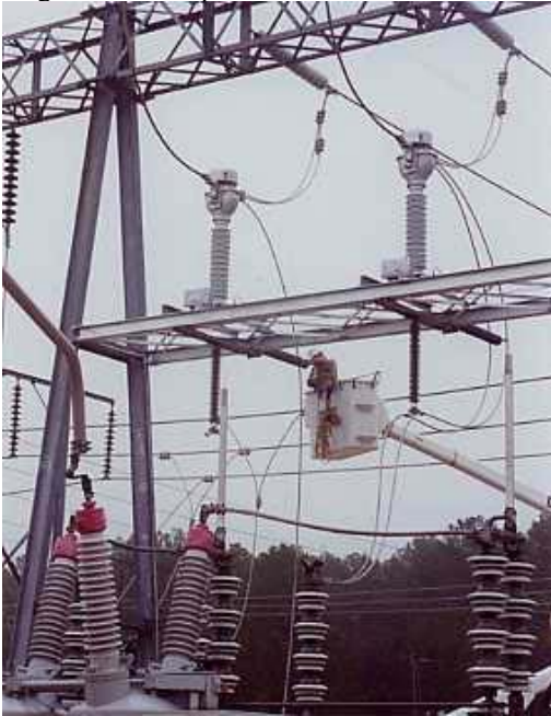
Figure 1. LCRA Transmission Construction crew installing an optical current transformer on overhead 138KV lines at a Sim Gideon Generator.
