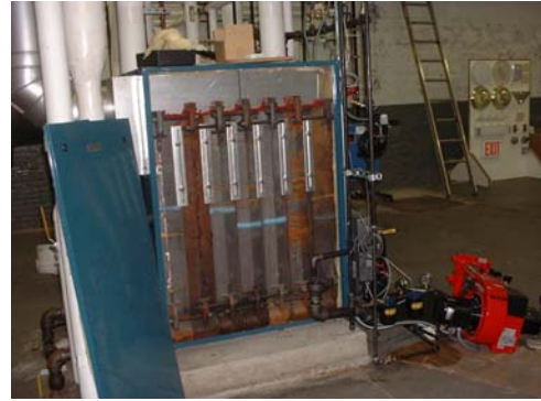
Figure 4 Boiler no.2 clean-out access for exercise
