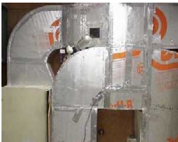
Figure 5. Photo of Desiccant Wheel Ducting on 2 1/2 Ton Air Handler.
