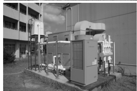
Picture 1. Outside Of HVAC&R Experimental Analysis System
