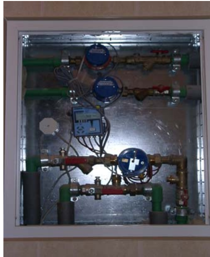
Image 5. Apartment's technical cabinet of the energy resource consumption register
