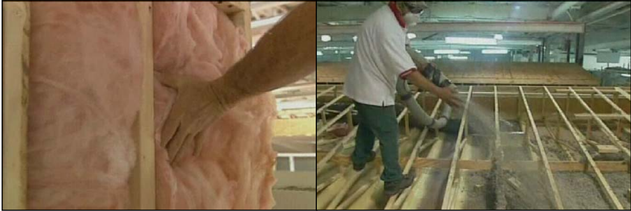
Figure 2. Manufactured unit R-19 wall insulation (left). R-26 blown ceiling insulation (right) Jacobsen, 2005.
