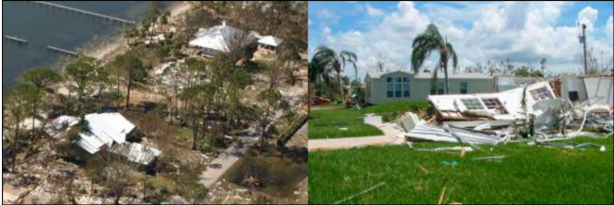
Figure 10. Pre-2002 FBC site-built homes destroyed, post-2002 FBC site-built homes intact (left). Pre-1994 HUD Code manufactured home destroyed, post-1994 HUD Code manufactured home intact (FMHA, 2004).
