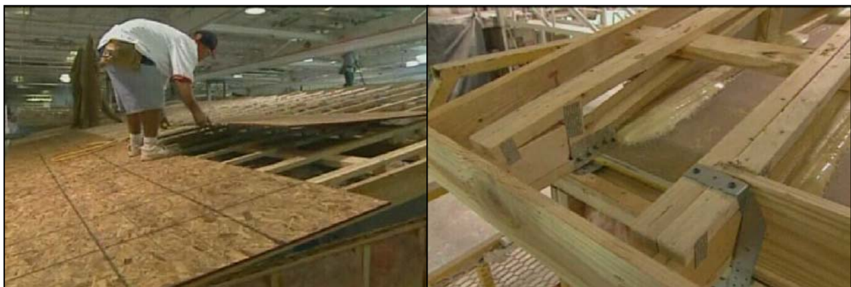
Figure 8. 13mm (1/2in) OSB roof sheathing (left). Doubled trusses within 1m (3ft) of each gable end with uplift tie-downs and straps (right) Jacobsen, 2005.
