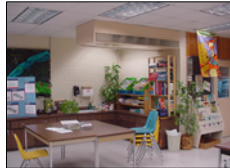
Figure 13. Air Handler in One of the Florida Elementary School #2 Classrooms
