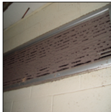
Figure 6. Main Return Grilles Behind Stage of
