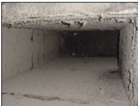
Figure 8. Dust in Return Duct after Outside Air Intake
