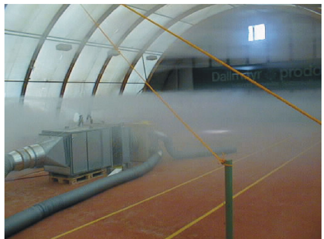
Figure 16 Verification of the forming of a stable thermal stratification by a smoke test
