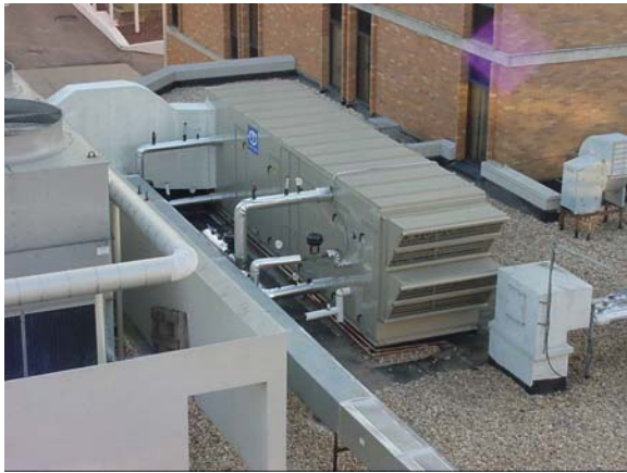
Figure 5: Desiccant unit showing side with pre-cooling and pre-heating coils
