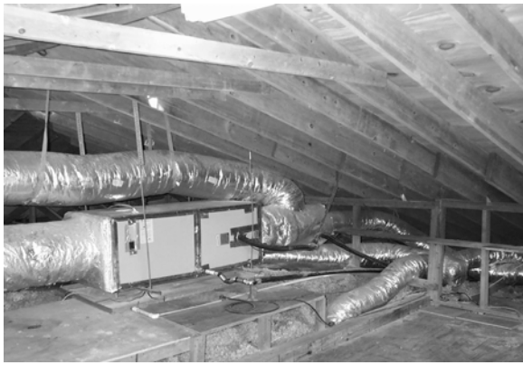
Figure 3. Site #199 showing attic air handler prior to retrofit.
