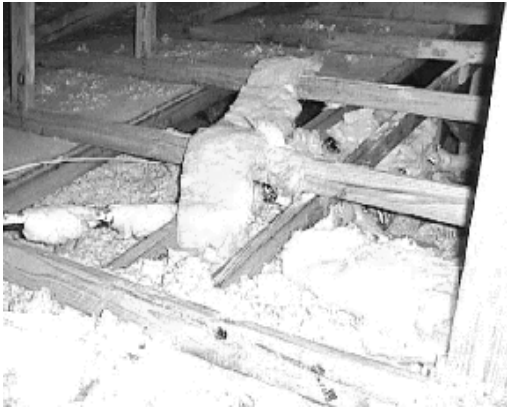
Figure 15. Uneven R-19 ceiling insulation at Site #126.
