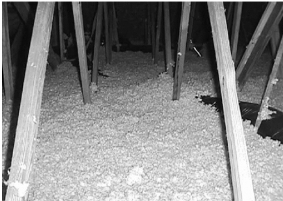
Figure 11. Excellent R-30 ceiling insulation at Site #72.
