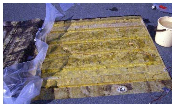
Figure 3. Wetting of a test roof of about 1000 m 2 . Initial moisture content in this test case was 20% of dry weight through the whole insulation layer. The roof dried out during one summer.
