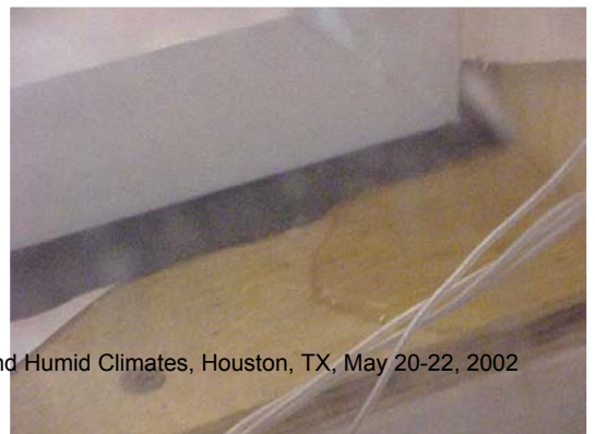
Figure 19: Water trapped by caulked sill flange collects at the bottom of window -- Wall C2.
