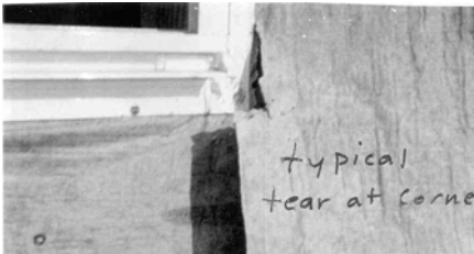
Figure 3: Damaged (torn) flashing
