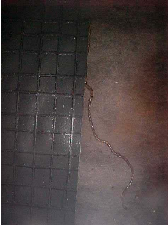
Figure 23: Water entering between the weather barrier and the jamb flashing.
