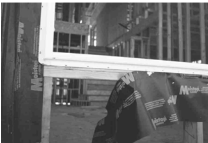
Figure 4: Partially detached flashing
