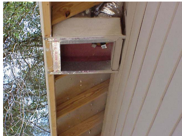
Figure 2 OA Intake Duct in Soffit
