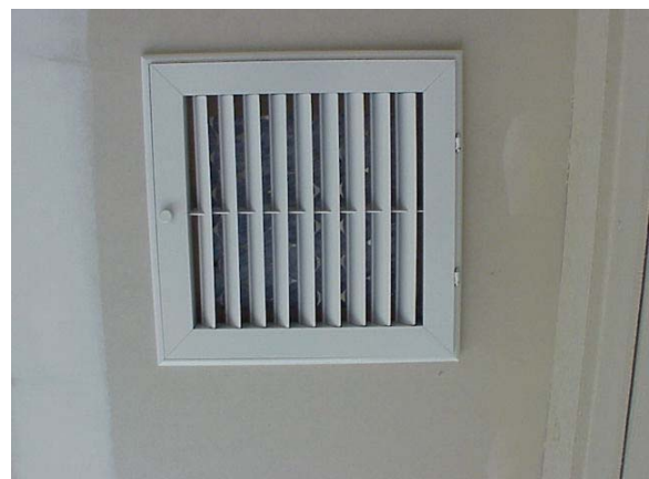
Figure 3 Filter Backed Grill Covering the OA Intake
