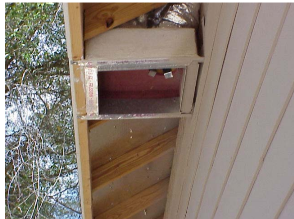
Figure 2 OA Intake Duct in Soffit
