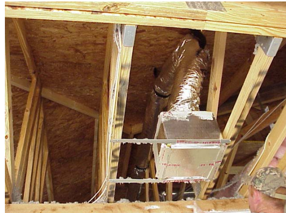
Figure 1 OA Intake Duct in Back Porch
