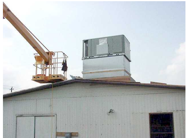
Figure 6. MODEL C Three Ton Rooftop Unit Installed on Storage Building
