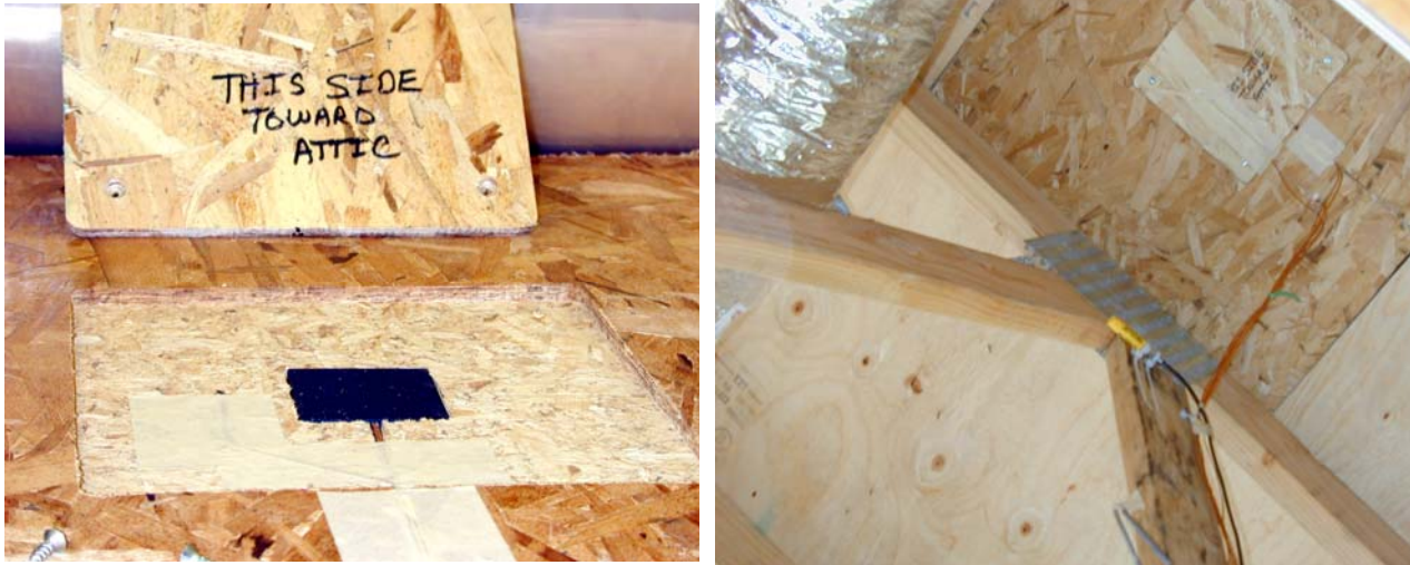
Figure 5. Heat flux transducer embedded in OSB guard and used to measure heat flow crossing roof decks of the demonstration homes with asphalt shingle roofs.
