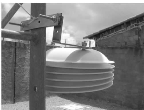
Figure 02 – Protection to the equipment
