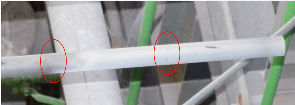
Fig. 2.23. Fouling sampling probe, with the TC0 (right) and TC1 (left) thermocouples
