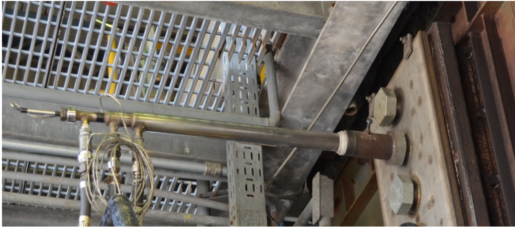
Fig. 2.22. The IFRF pyrometer inseted in port number 2
