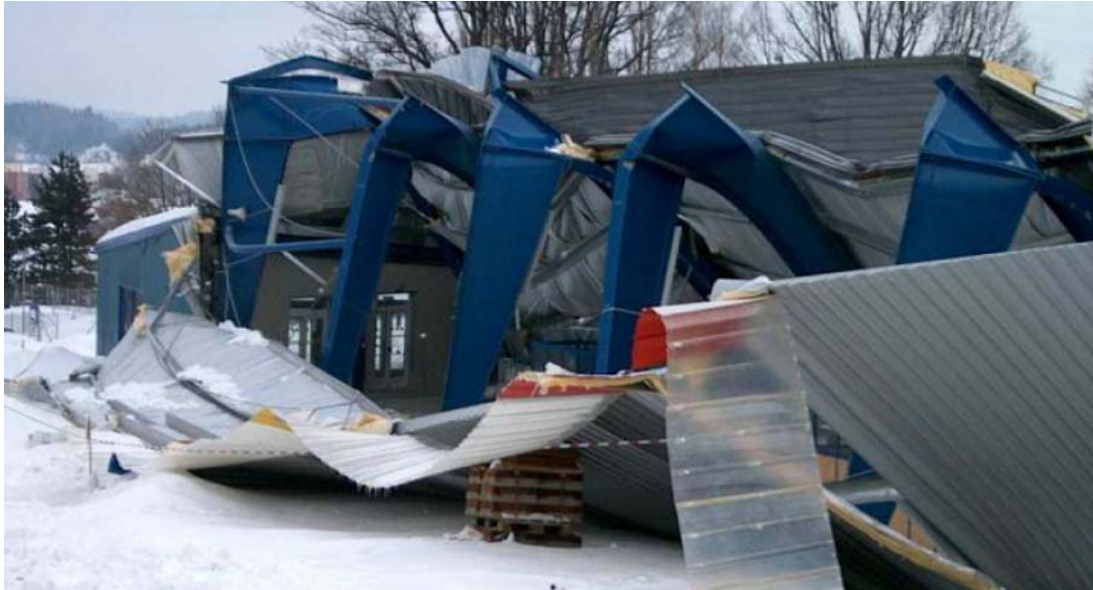
Figure 6.1: Collapse of a stadium
