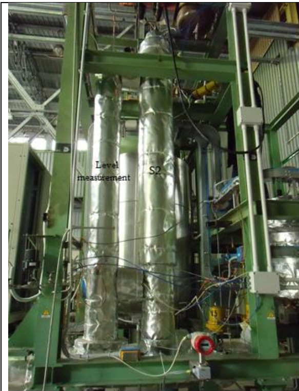
Figure 4.9 – view of S2 and level measurement system
