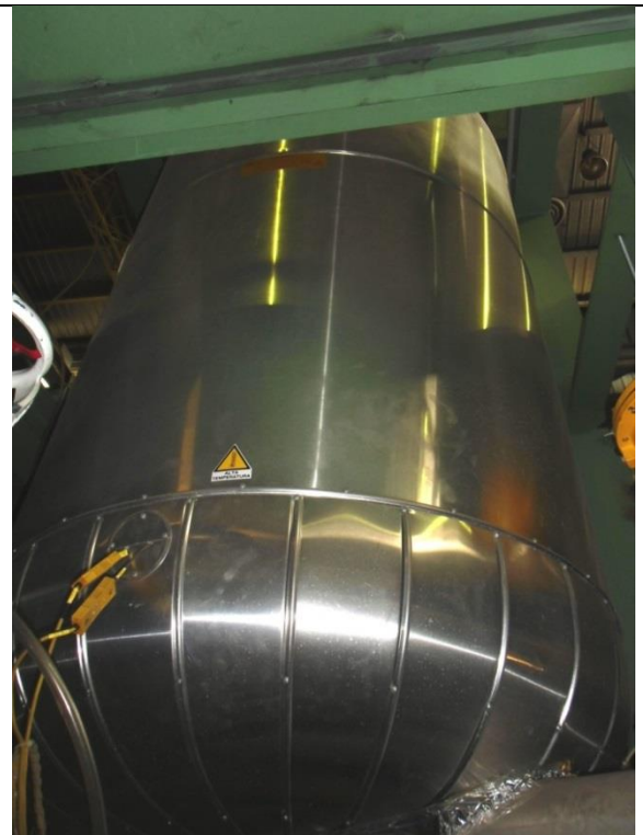
Figure 4.10 – view of S3 dump tank
