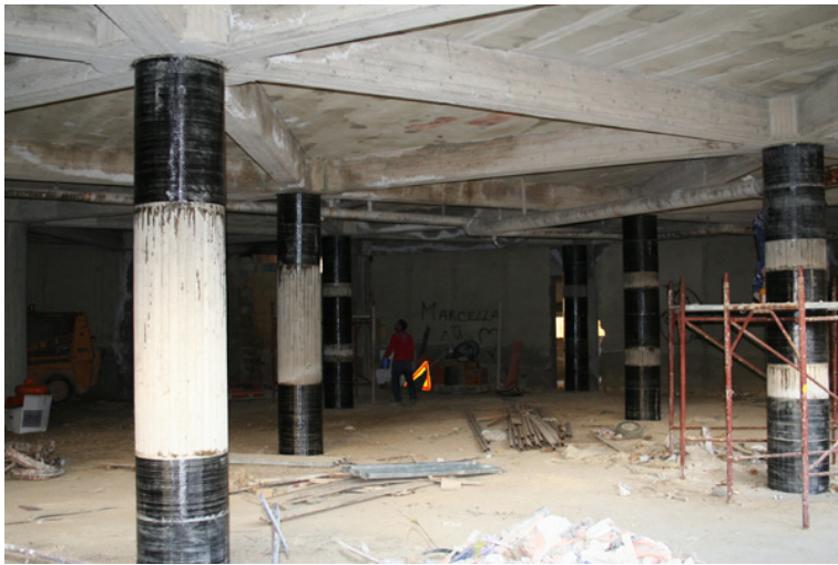
Figure 2.4: Strengthening of a circular reinforced concrete column using externally-bonded FRP wraps. (a) Confinement mechanism [3]; (b) Axial strengthening application.
